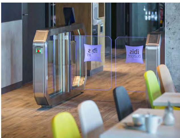
ACCESS CONTROL to the breakfast room
